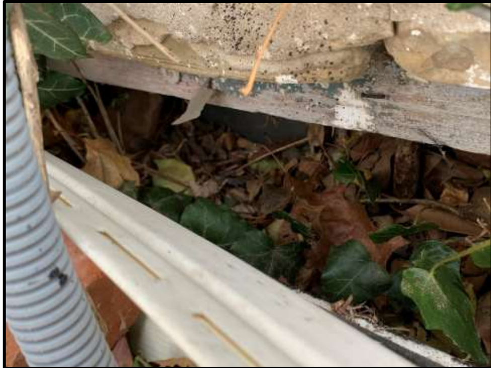
Image 11: Detail of wood frame basement window opening in west elevation (Photo taken on January 22, 2020)
