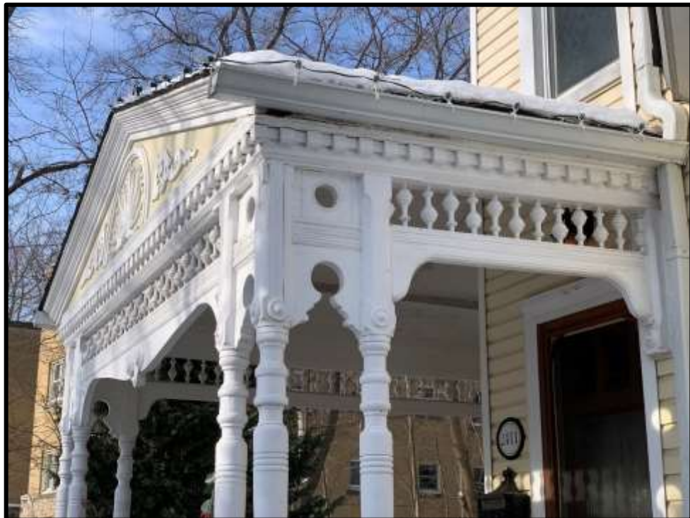
Image 6: Detail front door, covered porch and fine decorative woodwork (Photo taken on January 22, 2020; Facing East)
