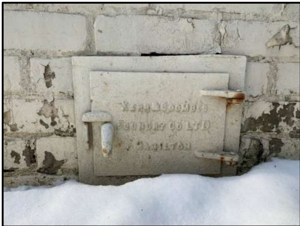
Image 22: East elevation detail of chimney access door "Kerr & Coombs Foundry Co. Ltd., Hamilton" (Photo taken on January 22, 2020)
