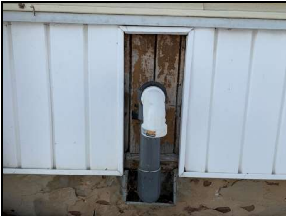
Image 20: East elevation detail of original wood cladding beneath vinyl siding (Photo taken on January 22, 2020)
