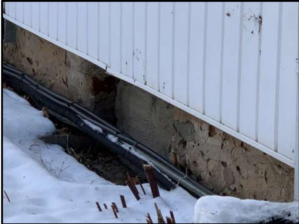
Image 19: East elevation detail of parged stone foundation and basement window opening (Photo taken on January 22, 2020)
