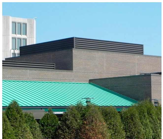
Screen rooftop equipment from view
