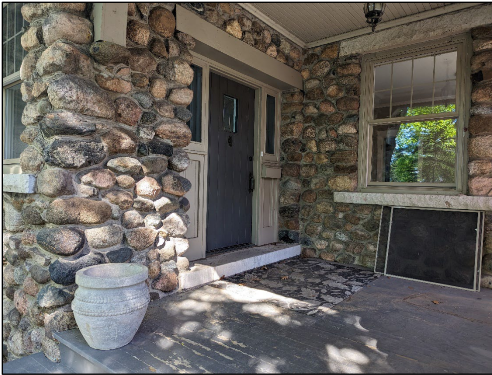
Figure 1: Front Window and Door Opening
